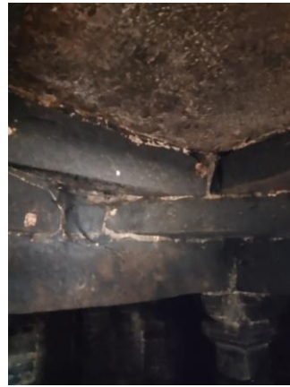
Soot deposition inside octagonal chamber
