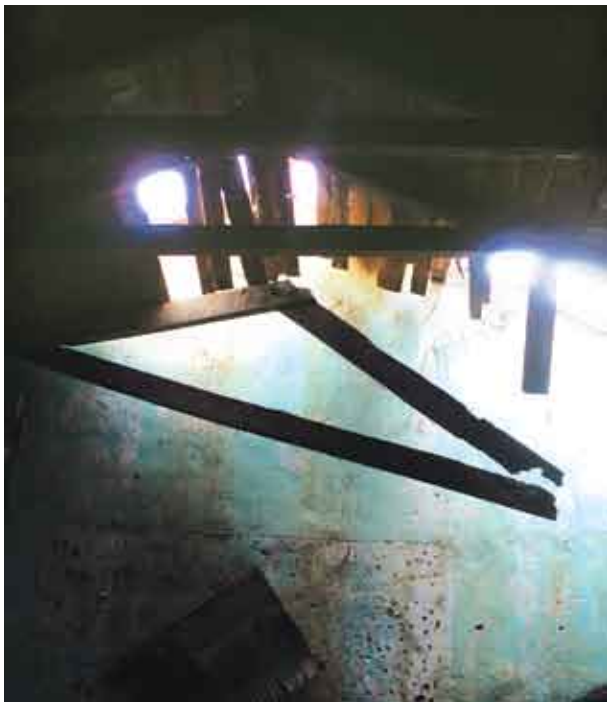
Broken rooftop in an Anganwadi Centre in Andhra Pradesh
